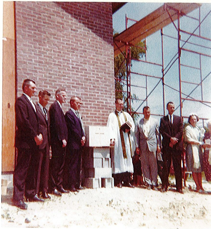
This color photograph shows the scaffolding on the east side of the church.
